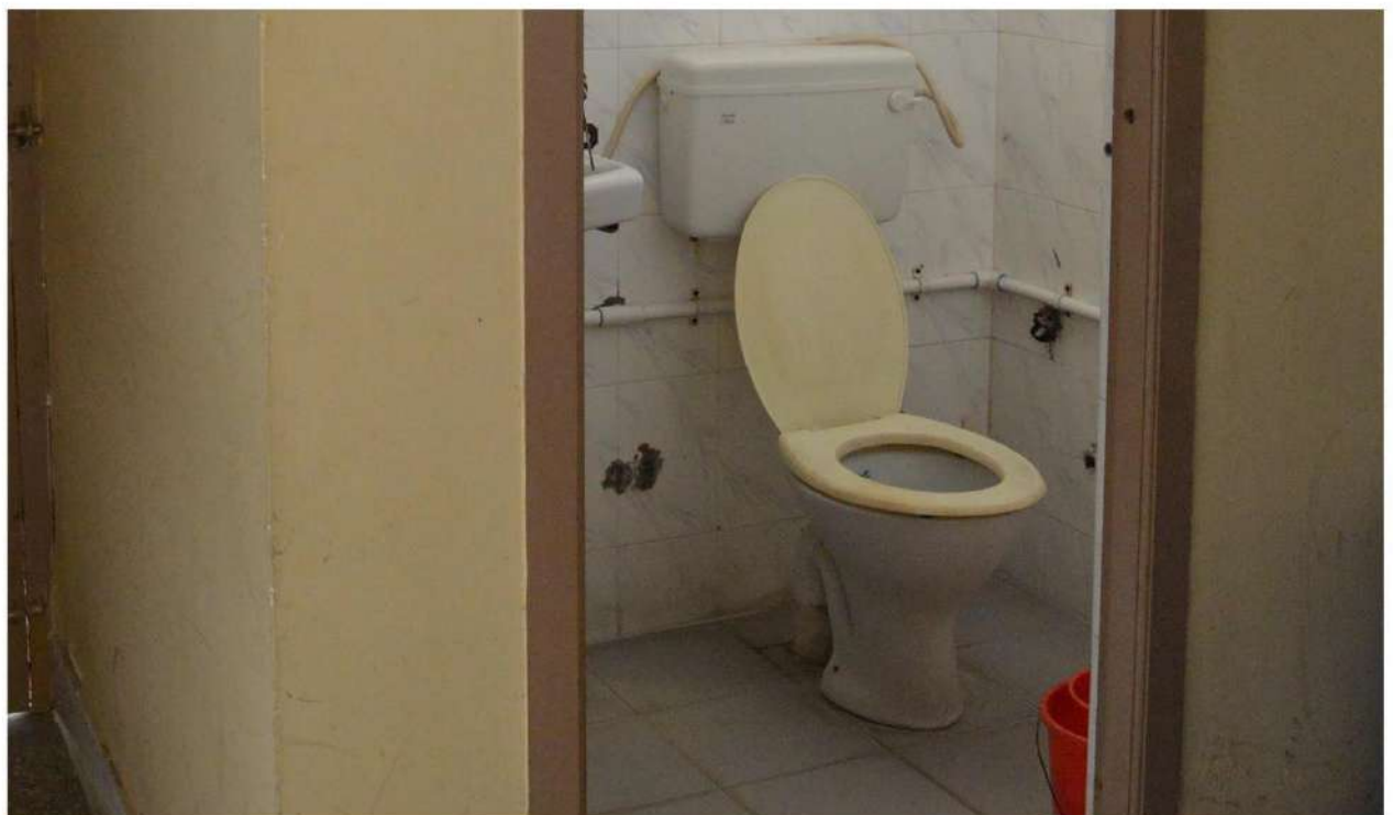
Special lavatory facility available for students at the computer Block
